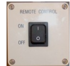
Main power switch
